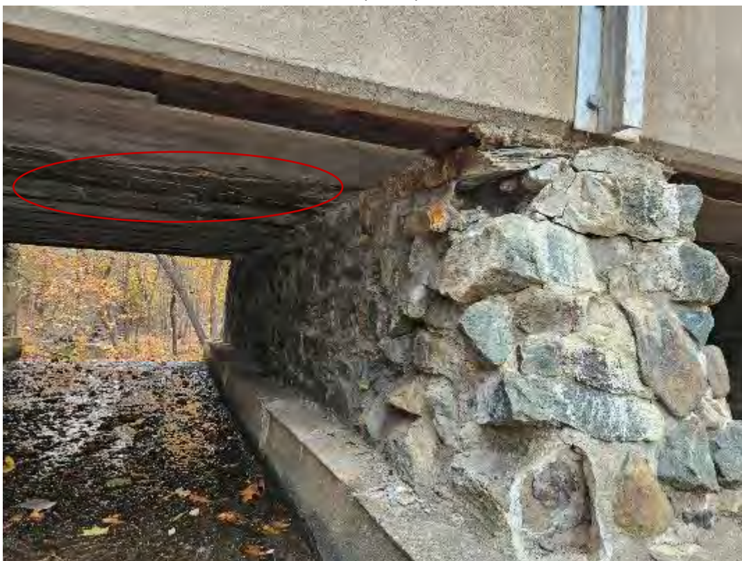
Photo 4: Bridge and abutment at spillway crest. Note erosion and exposed rebar under bridge deck.
