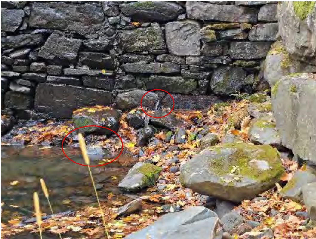
Photo 6: Location of seepage at base of dam.
