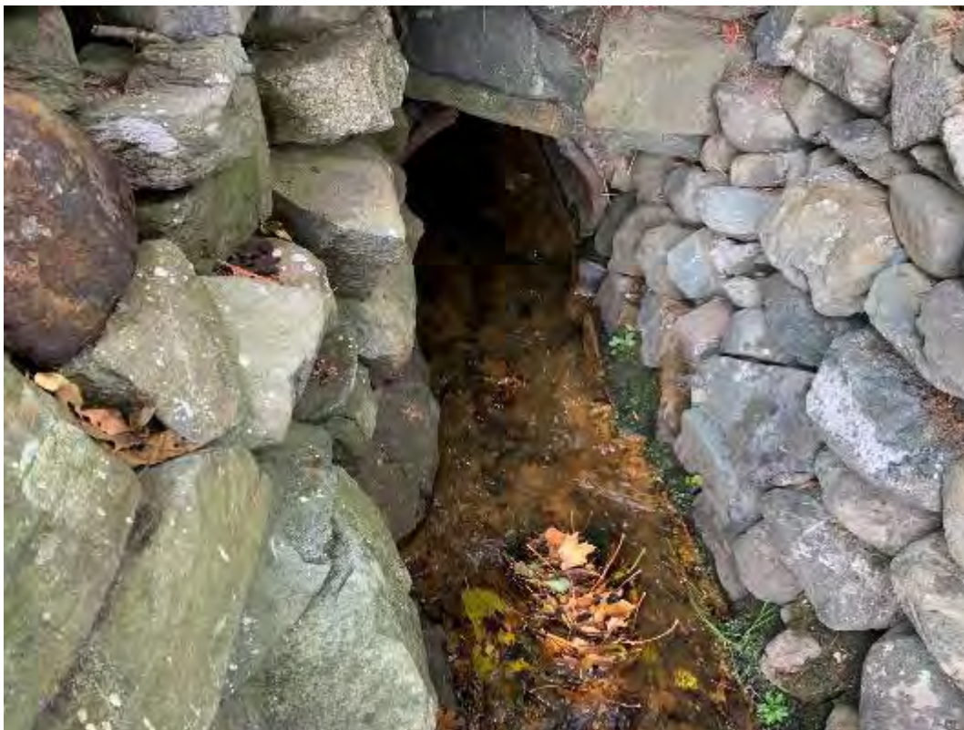
Photo 11: Deteriorating culvert section in stormwater ditch.
