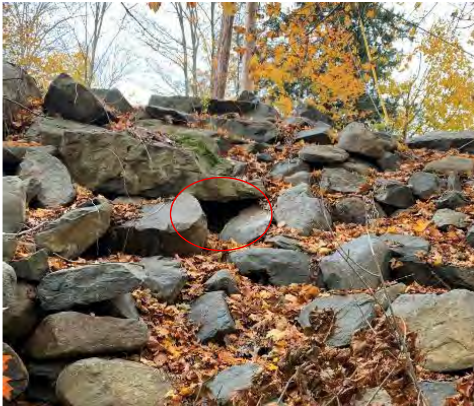
Photo 2: Voids in rock wall on downstream side of right embankment.
